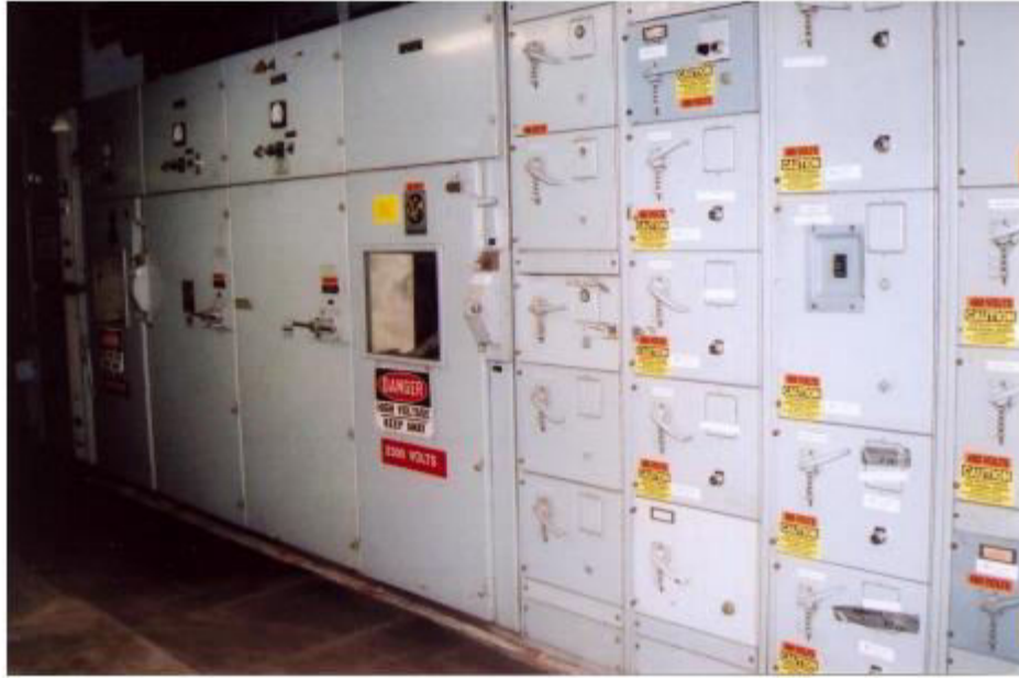
Figure 4. A sampling of the more than 300 electrical closets at a very large food warehouse in New Jersey.
