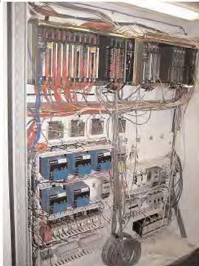
PLC remote I/O racks, burner controls, numerous AC "ice cube" relays
