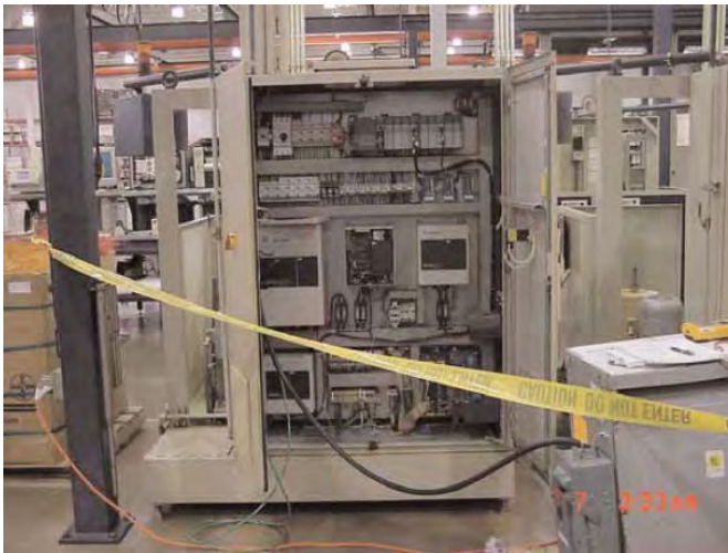
Horizontal Line Take-Up Drive Cabinet
