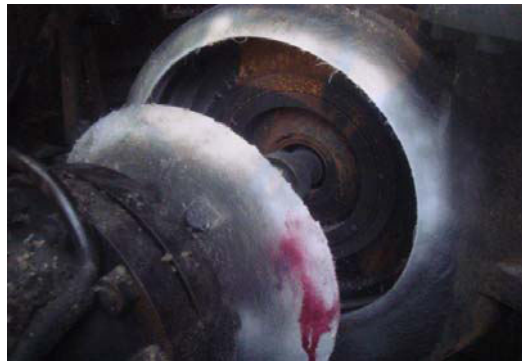
Casing plate of crude booster cut circumferentially by rubbing action of impeller.
