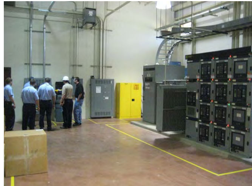
Team Examines Switchgear and EDP panels in Bldg 801 Mechanical Room
