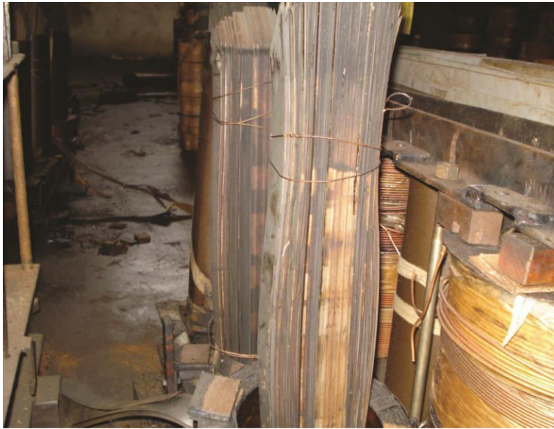
Fig. 5: Core insulation failure...
