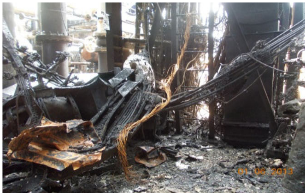
Burnt Instrument & Electrical cables
