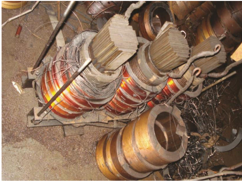
Fig.6: Failure due to paper block shrinkage...
