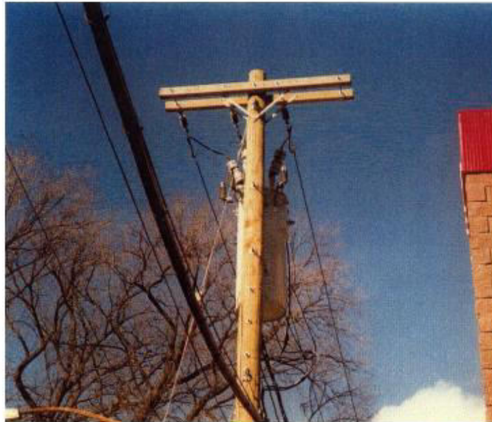
Figure 2. Telephone pole with 3-phase 13,000 Volt power cable near building (right) where accident occurred.
